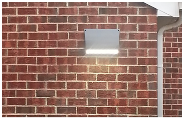
Exterior-Installed LED Lights
